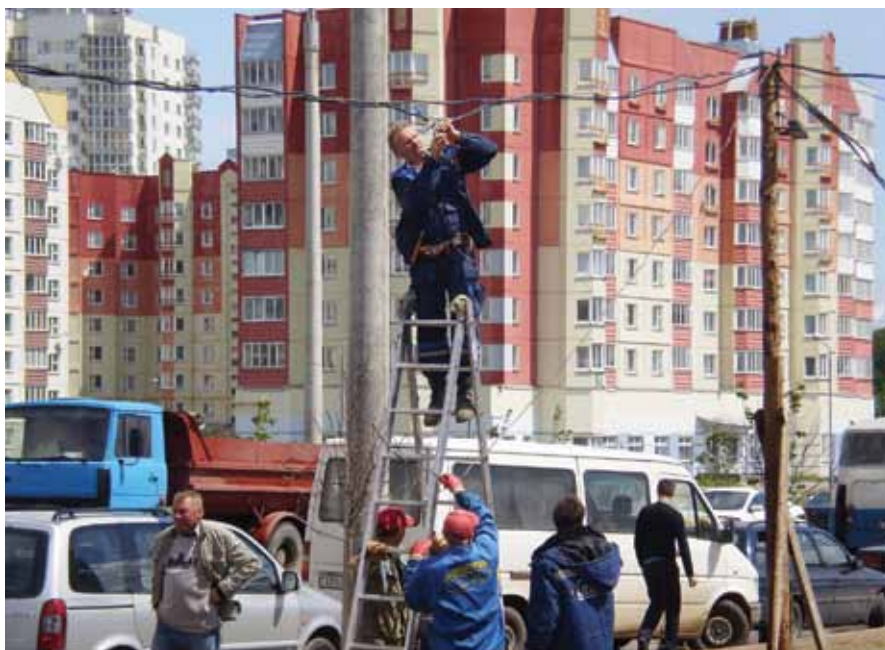
Inobservance of occupational safety rules: workers work without helmets.
