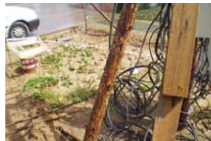
Disorderly electricity network, open wires.
