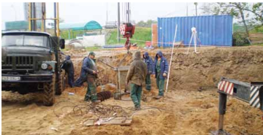
Workers work without helmets.
